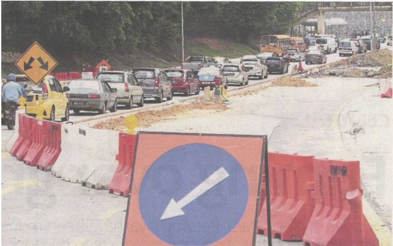
Utility works along Jalan Utara, Petaling Jaya, have reduced a six-lane road to one lane. — Photos: AZLINA ABDULLAH/The Star
